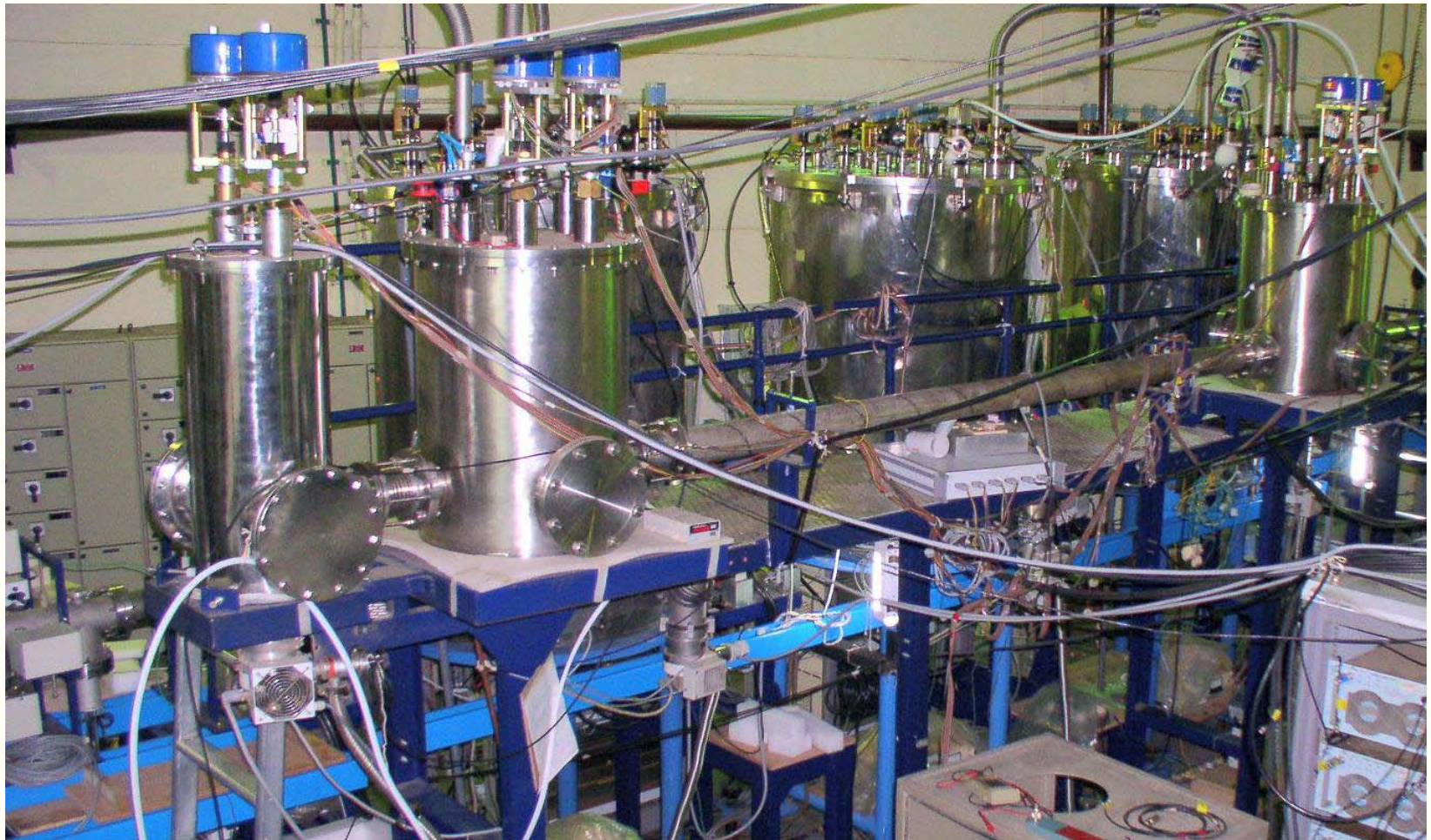
Cryostat modules housing the resonators with liquid He distribution box
